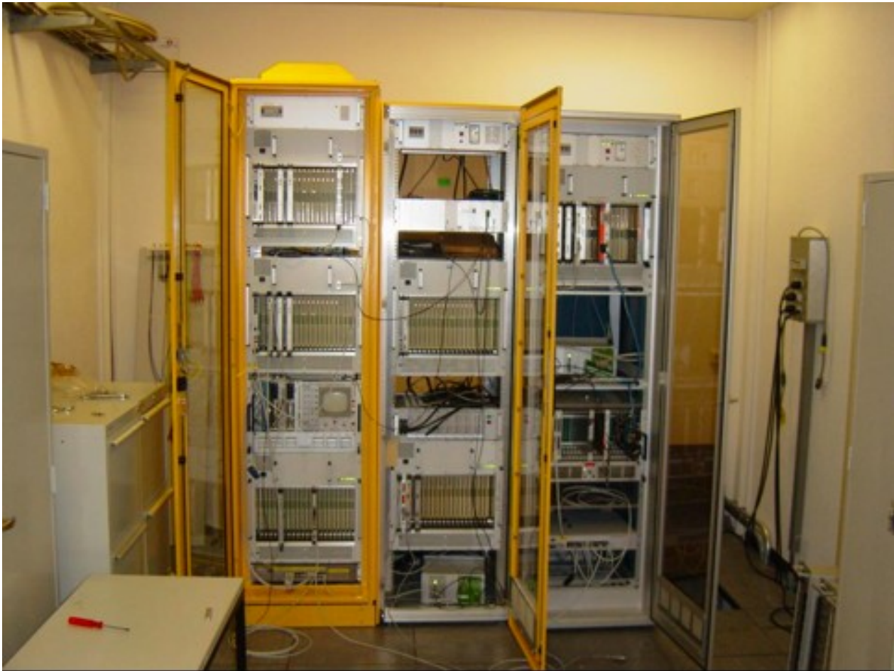
Figure 1.5: Device control layer - VME crates
