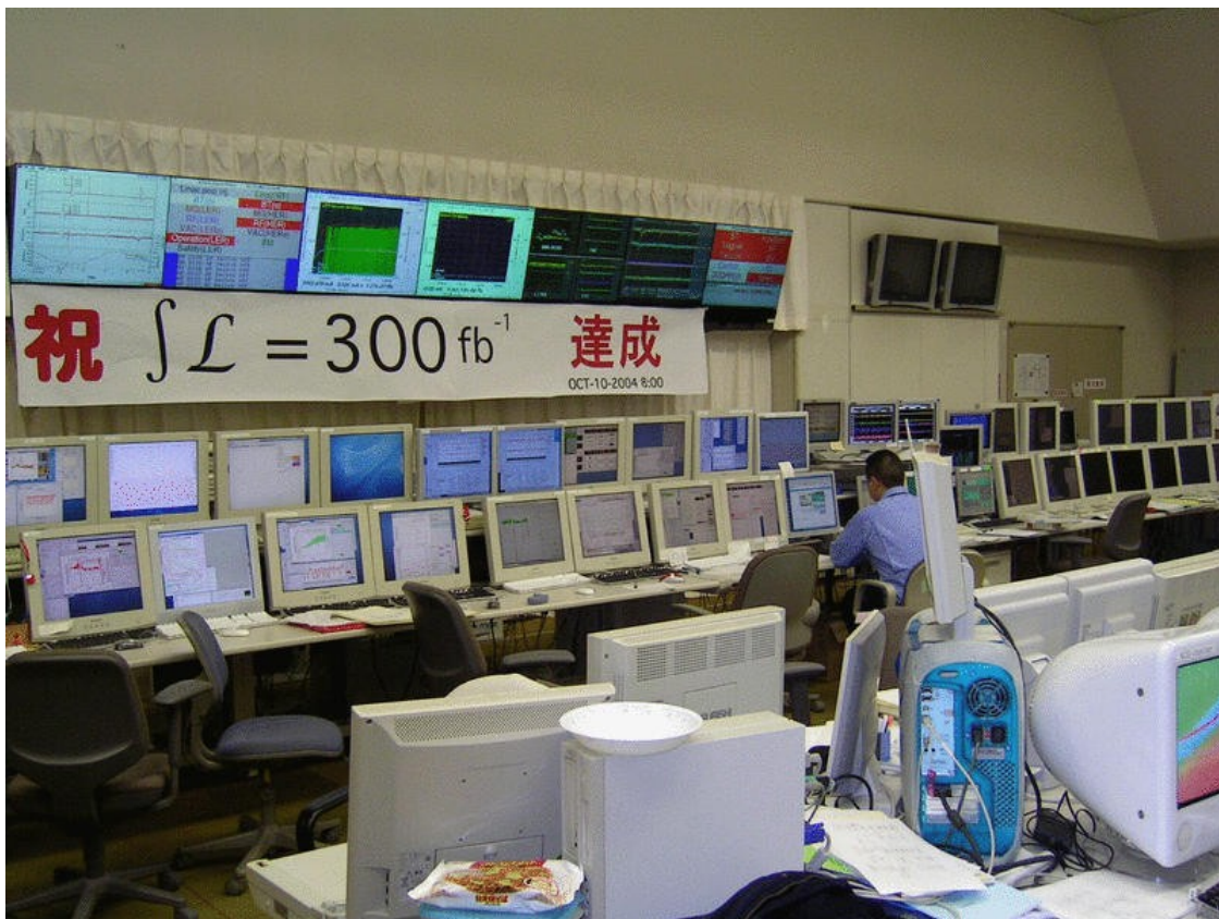
Figure 1.3: Presentation layer - operator consoles in KEKB control room
