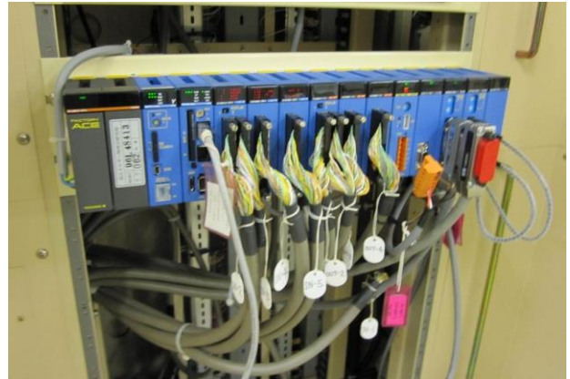
Figure 5: FA-M3-based IOC for vacuum control. From left to right, a Power Supply, a normal sequence CPU an F3RP61 CPU and I/O modules.
