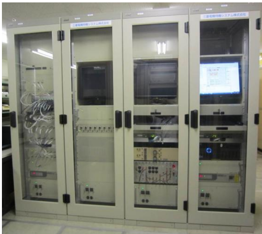
Figure 4: Digital LLRF system. FA-M3-based IOC is on the other side of the leftmost rack.
