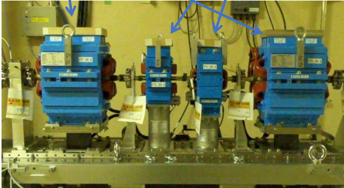
Typical magnet set at 3-5 sector of LINAC
