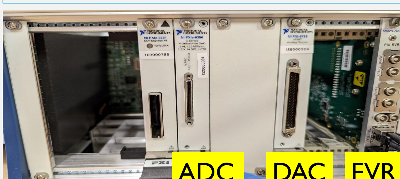
PXIe chassis and modules
