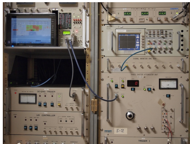
Figure 3 b): The photograph of a new KLY control system.
