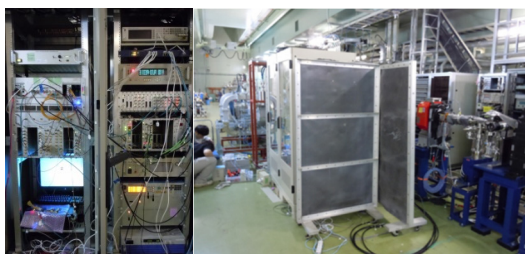
Figure 4: LLRF system for Capture Cryomodule configured inside STF Accelerator tunnel.
