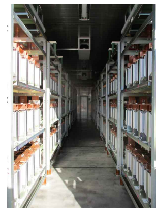
Figure 6: Metal racks installed in the marine container.
