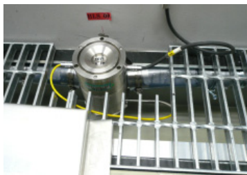
Figure 6: HLS in the tunnel pit.
