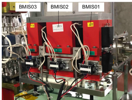
Figure 3: Chicane magnet installed in the cERL.
