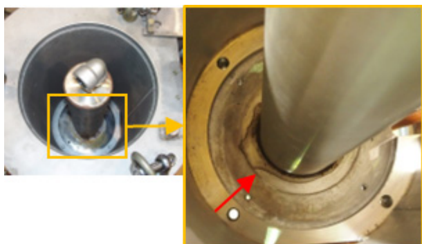
Figure 7: Water Leak point.
