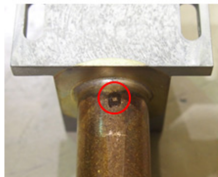
Figure 3: Cooling Water pipe pinhole.
