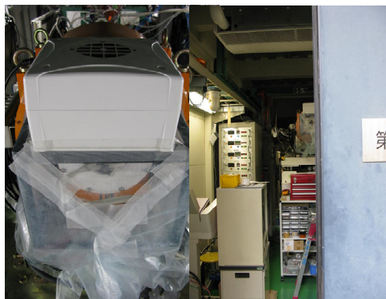
Figure 4: Simple air purifier for Gyrotron.
