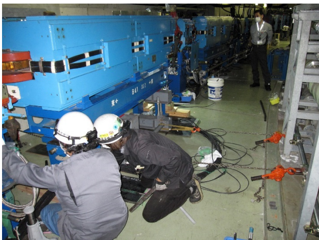
Figure 5: The pulling work of a bending magnet to install a vacuum chamber.
