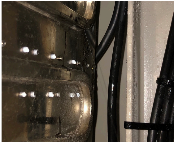
Figure 10: Leakage of cooling water of the cooling plate of transistors in the power supply for the sextupole magnet.
