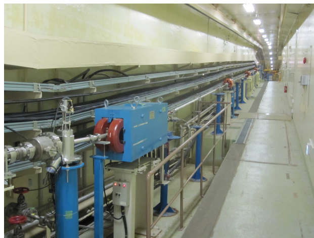
Figure 1: Photo of the PF-BT. The PF-BT is a 2.5 GeV beam transport line with a total length of about 170 m and connects the end of the LINAC located underground to the injection point of the PF-ring located at ground level.
