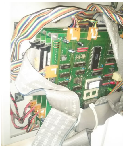
Figure 5: Photograph of personnel key system control board.
