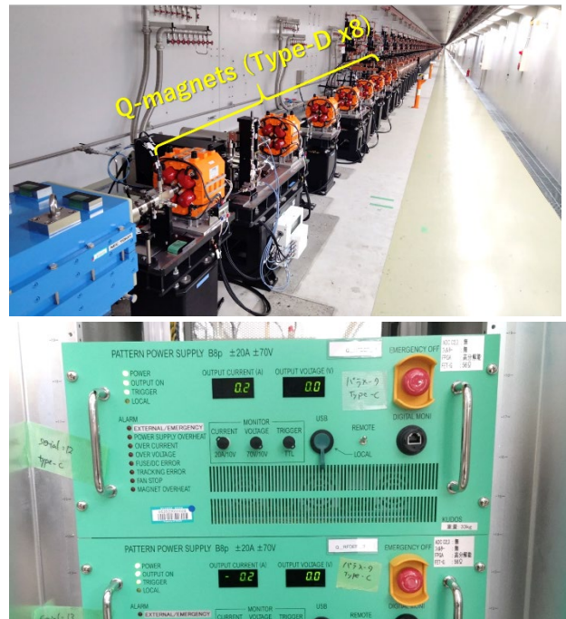
Figure 6: Photographs of the installed Q Type-D magnets in the matching section (Upper), and the pattern PSs (Lower).
