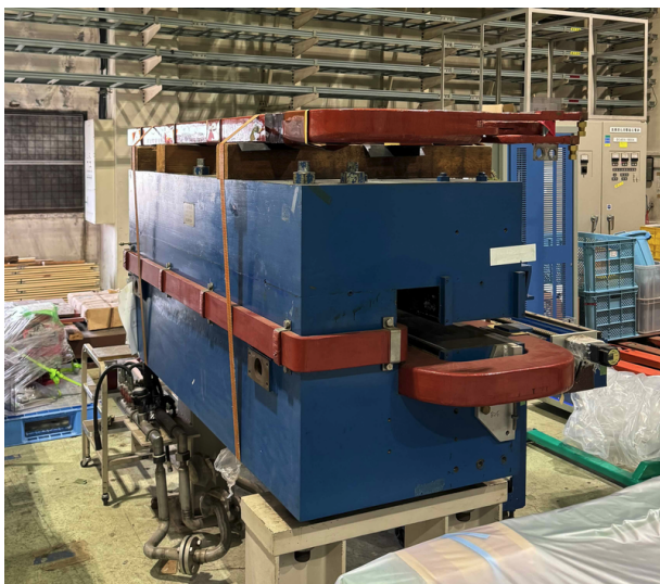
Figure 13: The broken coil placed on the return-yoke of # 13 bending magnet.
