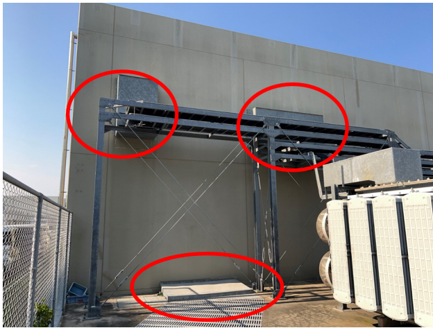
Figure 5: Power cable penetration points (in ovals in the figure).
