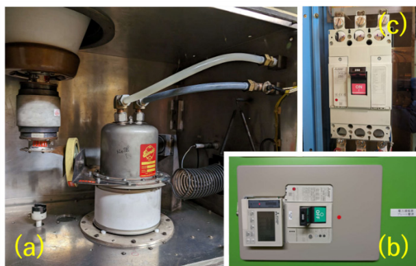
Figure 6: Replaced devices for AVF. (a) Vacuum tube, (b) ELCB, (c) MCCB.
